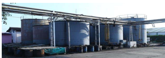
Solvent Extraction Plant and Oil Refinery at Khandwa (Khandwa Oils Unit - I)
