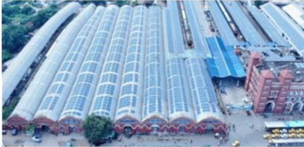
3 MW Rooftop Solar plant at Howrah Railway Stations
