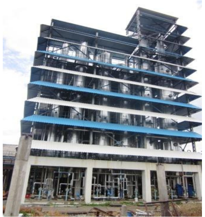
Multi Purpose Vacuum Distillation Plant
